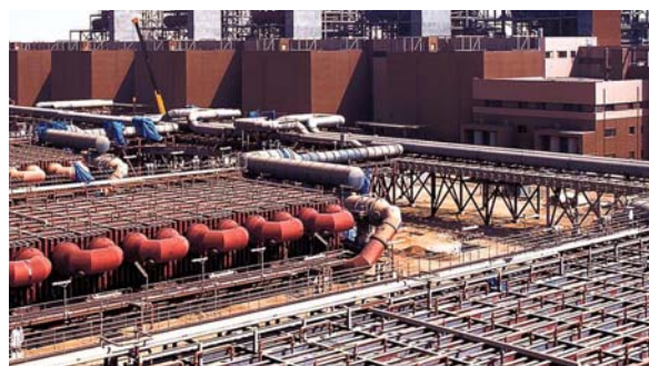
Desalination Plant (Resource : Doo San heavy industries)
